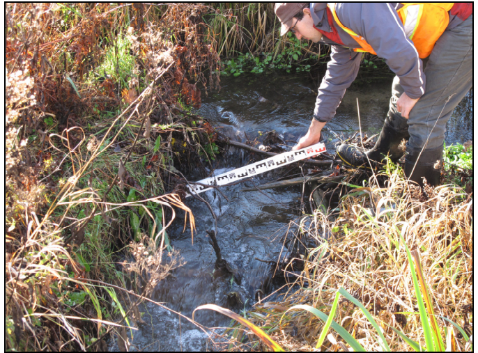
Photo 4: Reach 2 - Refer to Figure ERSN 1 for location of shot. Series of Several headcuts were found
