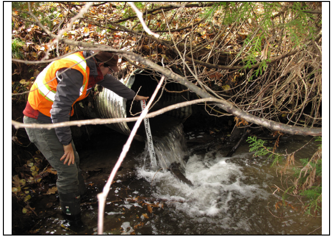
Photo 2: Reach 2 - Refer to Figure ERSN 1 for location of shot. Perched culvert.
