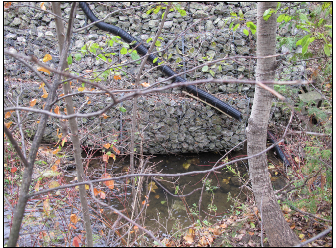
Photo 8: Reach 4 – Refer to Figure ERSN 1 for location of shot. Slumping gabion basket with water flowing underneath it.
