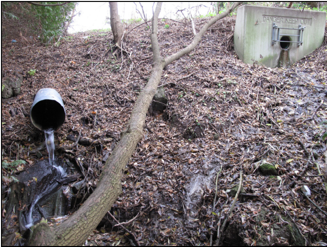
Photo 11: Reach 10 – Refer to Figure ERSN 1 for location of shot. Several Perched Culverts.
