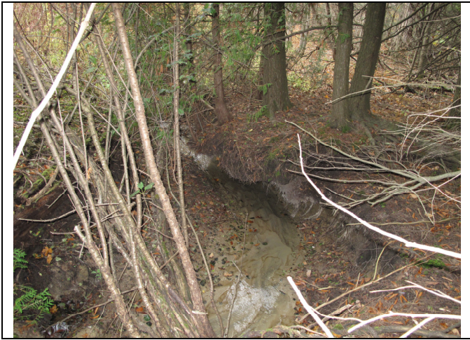
Photo 13: Reach 12 – Refer to Figure ERSN 1 for location of shot. Some undercut sections and erosion noticed right off of West Turner St
