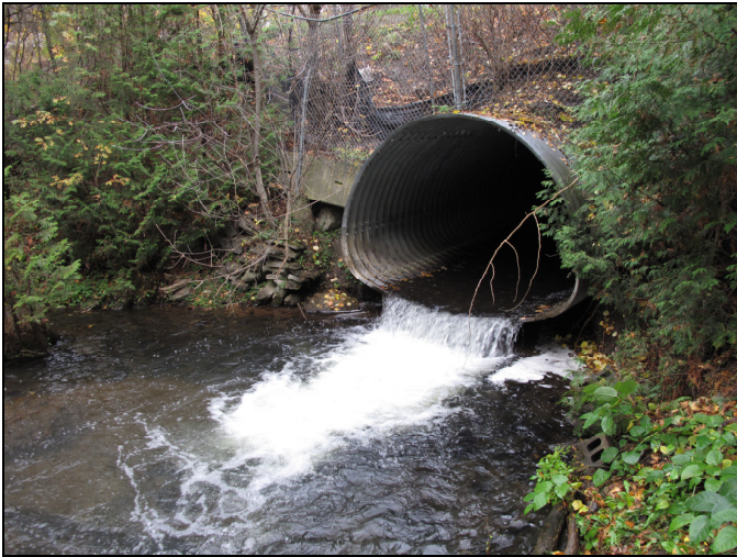
Photo 15: Reach 16- Refer to Figure ERSN 1 for location of shot. Perched Culvert.
