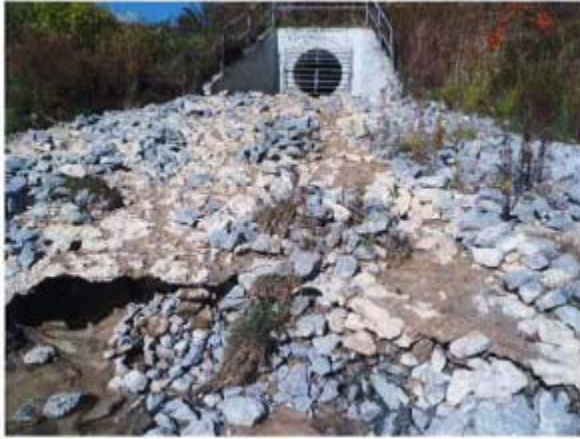
East inlet headwall, Erosion protection
