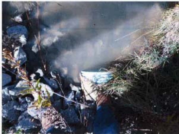
Outlet Structure, Quality Control Pipe
