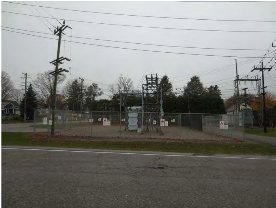
Photo 13 – Neighbouring land to the west: electrical substation (looking west across Donland Lane).
