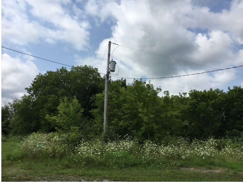
Photo 7: Hydro pole with transformer across the road from the storage shed.
