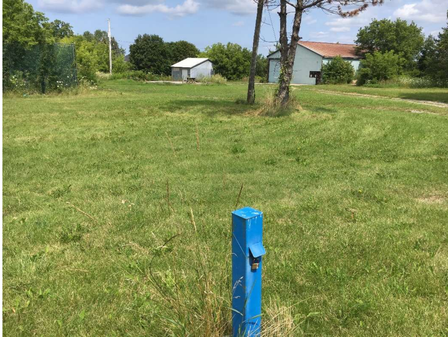
Photo 17: Groundwater monitoring well installed near former ASTs on west side of driveway.
